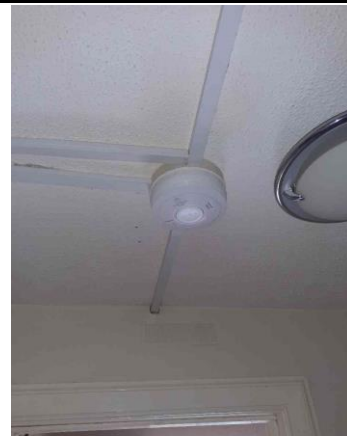
Smoke - Hall (Floor 1)
