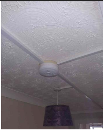
Smoke - Hall (Floor 1)
